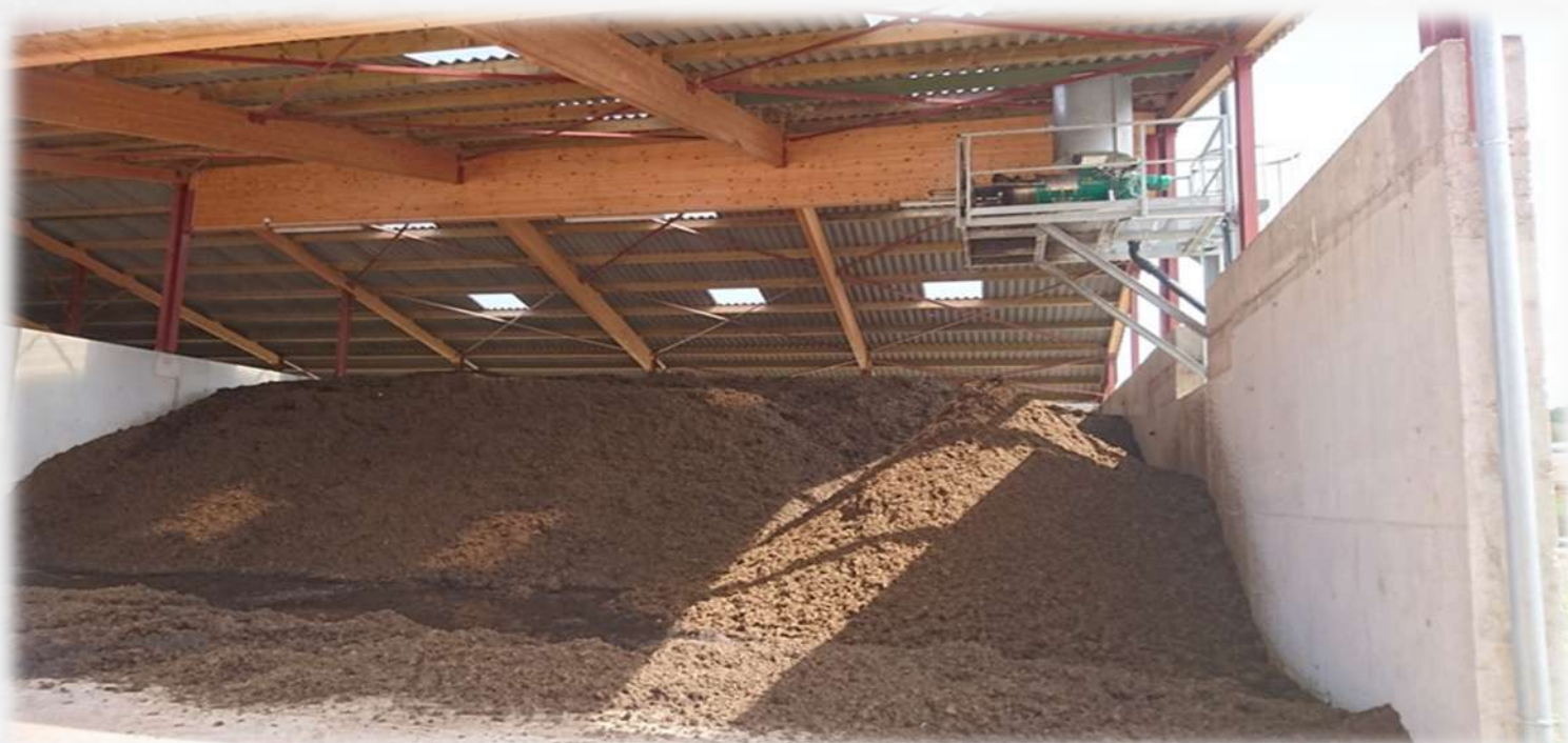
Stockage digestat solide SASU Biogaz Energie
